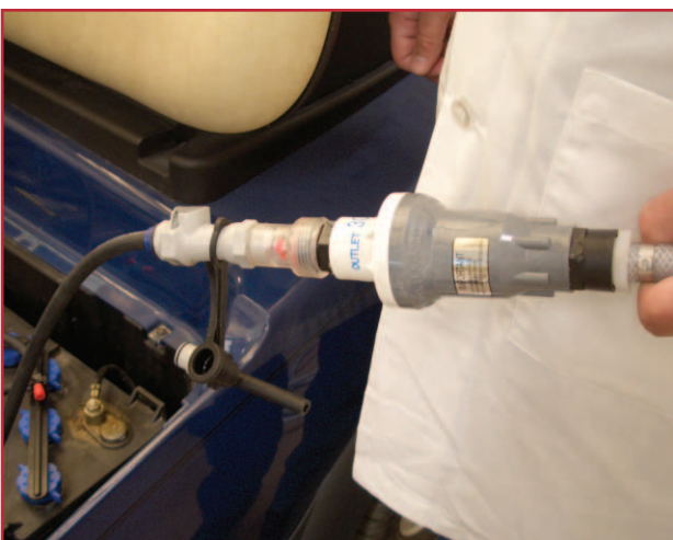
The battery is watered by connecting a hose from the facility water supply. The hose end assembly includes a pressure regulator and flow indicator.
